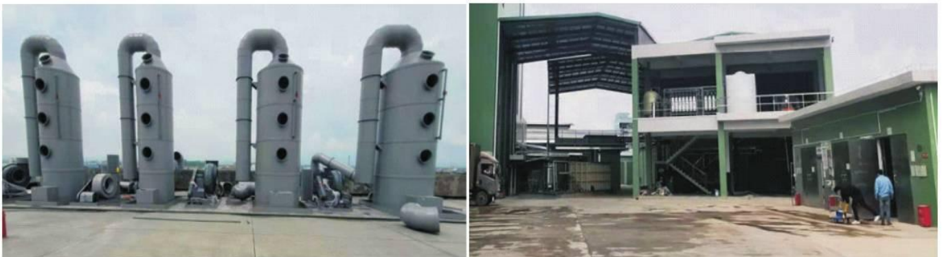
SEWAGE TREATMENT PLANT, 100% COVER DISCHARGE DEMAND FROM PRODUCTION CAPACITY.
